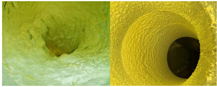
Figure 3. Major build-up (left) vs minor build-up (right) inside ducting.
